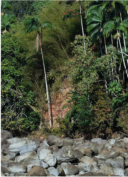
Erosion in Wailuku stream bank
