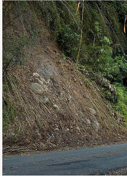
Erosion near Honolii bridge
